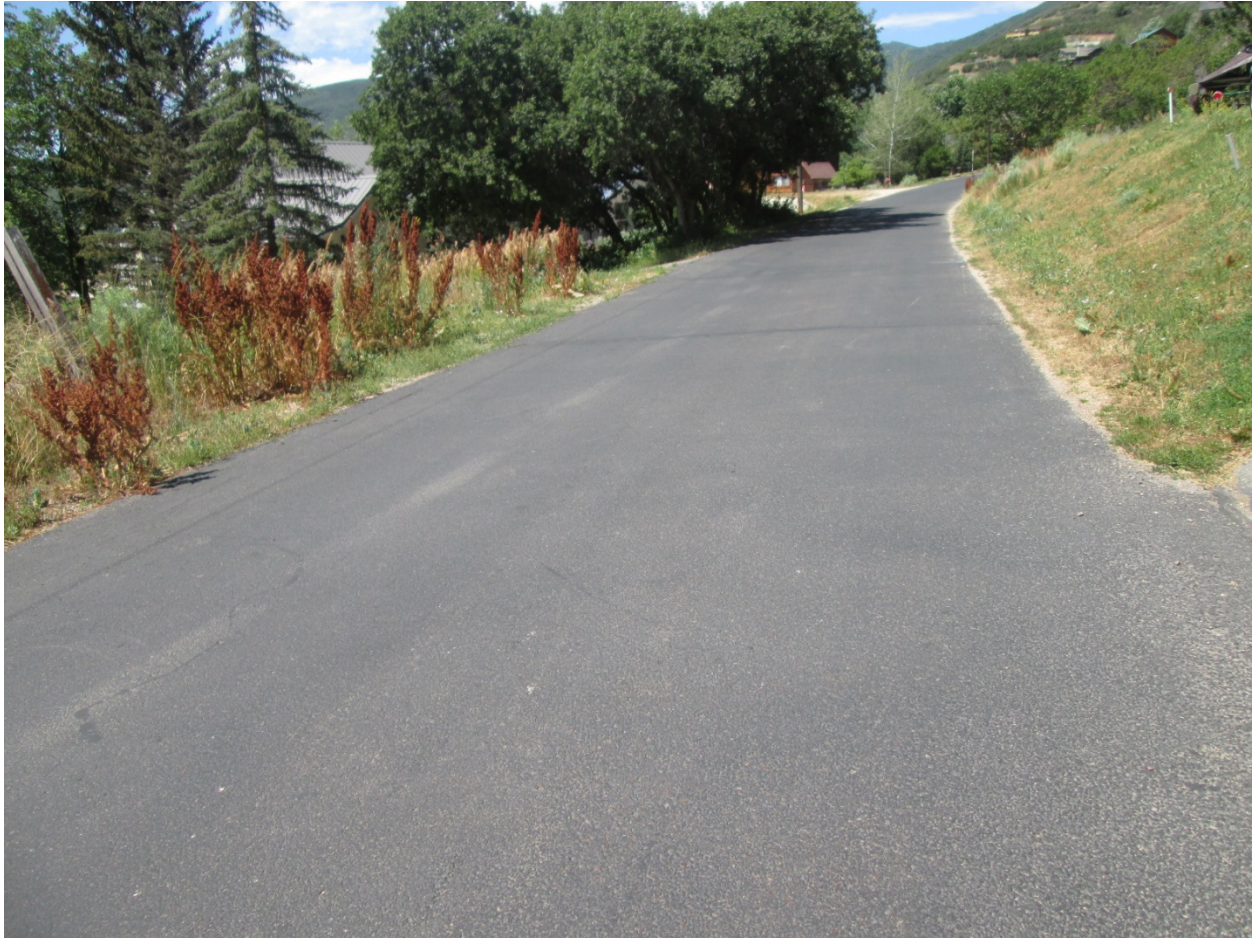
Photo 2. Good Condition – Interlaken Dr from Interlaken Dr to Luzern Rd (RSL = 10 years)
